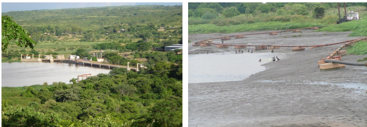
Figure 2: The Water intake dam at Nkula Falls on the Shire River (left); heavy siltation (right)
